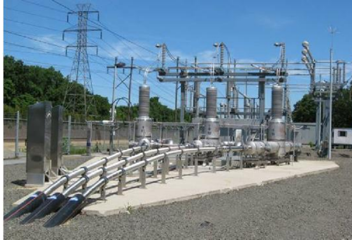
World's longest HTS cable (at that time) successfully energized on April 22, 2008
