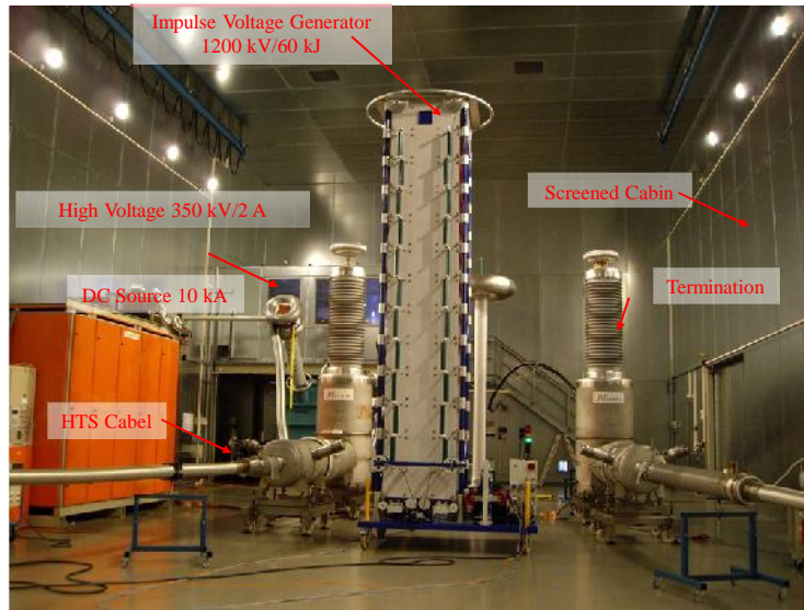
138 kV, 2400 A, 30 m Prototype in the test field in Hanover
